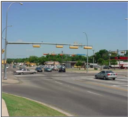
Horizontal traffic signal, attached to mast arm, cobra head light street light
