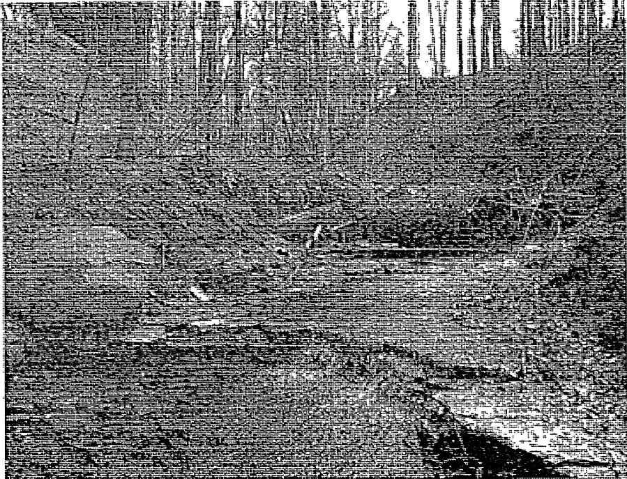
Gabion basket placed for grade control on limestone/shale bed in Northern tributary; facing upstream on east side of Thurston. Incised channel with steep water surface slope and erosive banks.
