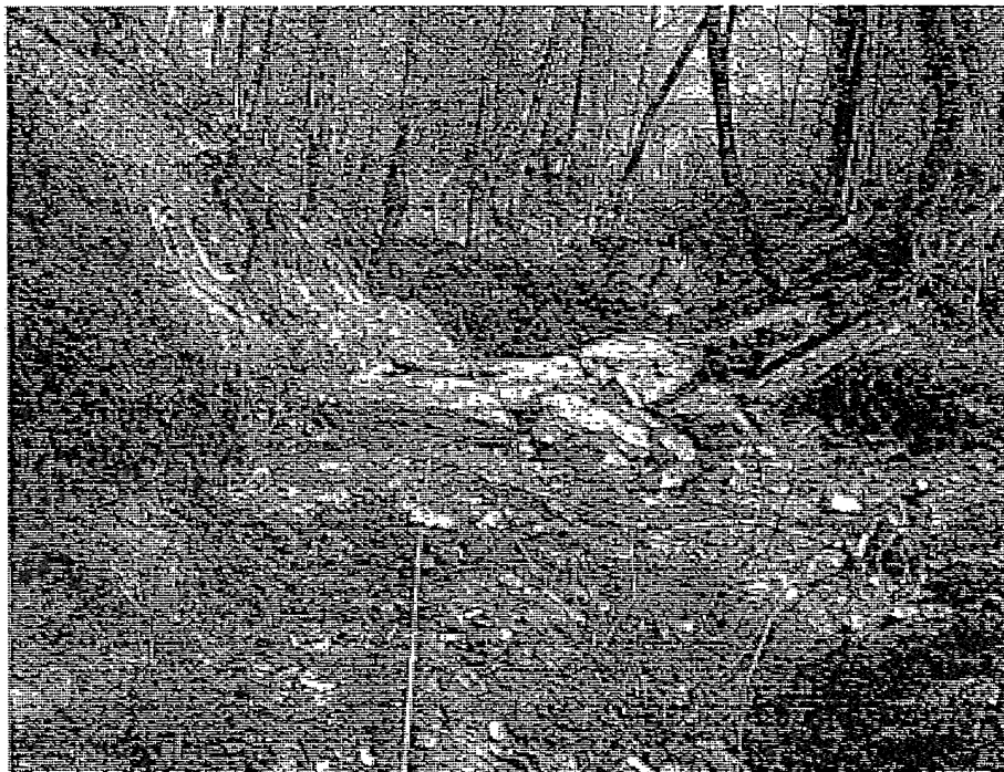
Facing upstream in highly unstable tributary below the Oneida Street culverts but above the outfall to the Sauquoit Creek. Proposed Step Pool Storm Conveyance project incorporating stormwater storage, grade control and habitat improvements.
