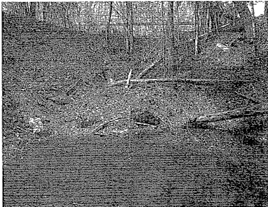
Facing downstream toward the upstream invert of the Brantwood culvert which becomes easily blocked and has resulted in road flooding in spite of the elevation difference between the pipe and the road. Propose to right size the culvert.
