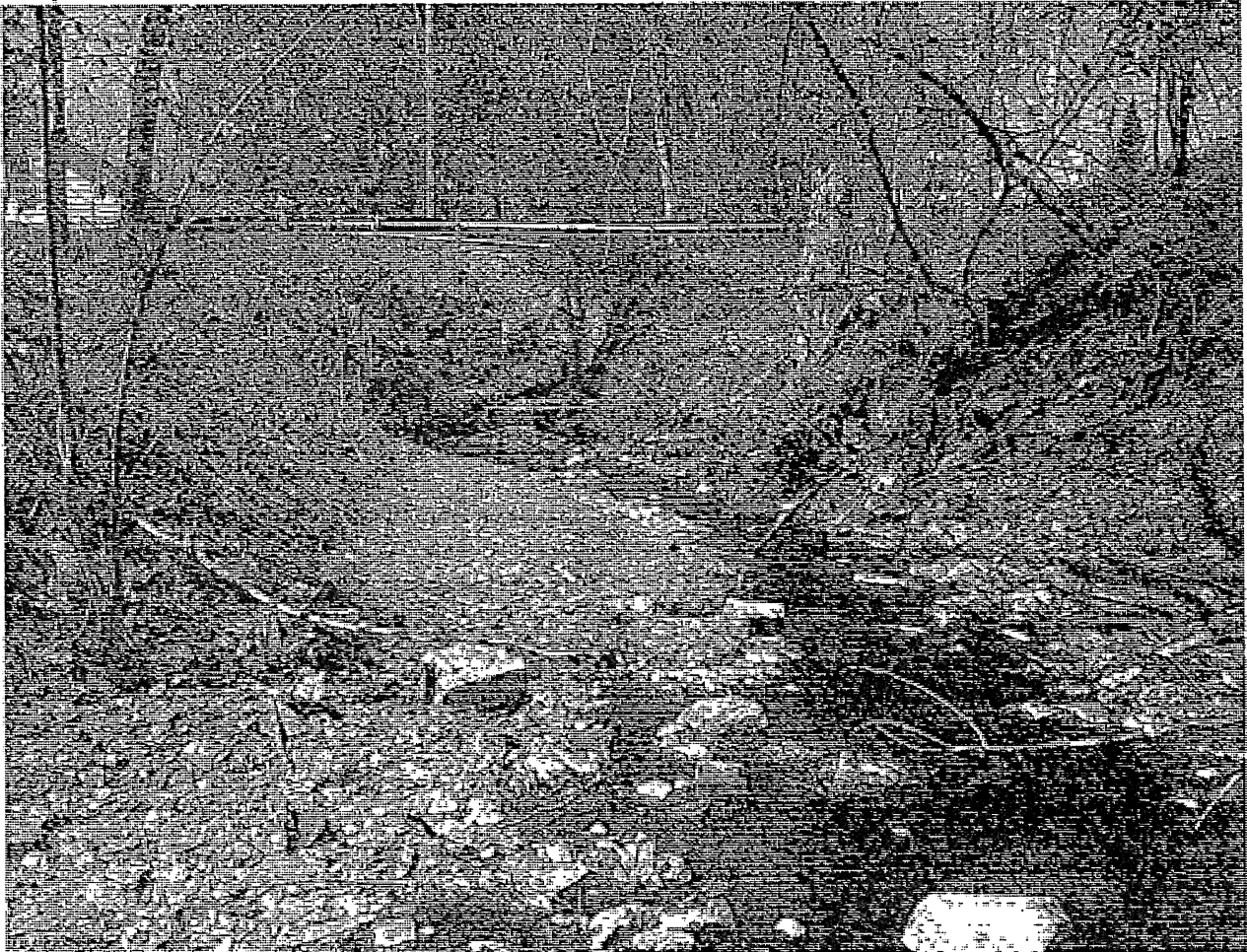
Facing downstream toward Oneida Street culvert. Note that only the northern culvert is visible as the southern culvert pipe is entirely blocked at the upstream side. The culverts are twin 2.2' smooth bore pipes.
