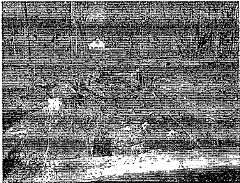
Southern tributary channelized in concrete armored channel in lawn downstream of Thurston. Note that between this channel and Thurston (in the upstream direction), the channel is enclosed in a corrugated metal pipe. The landowner had provided verbal permission in May of 2018 to daylight the enclosed channel but there is nothing officially documenting this as of this writing.
