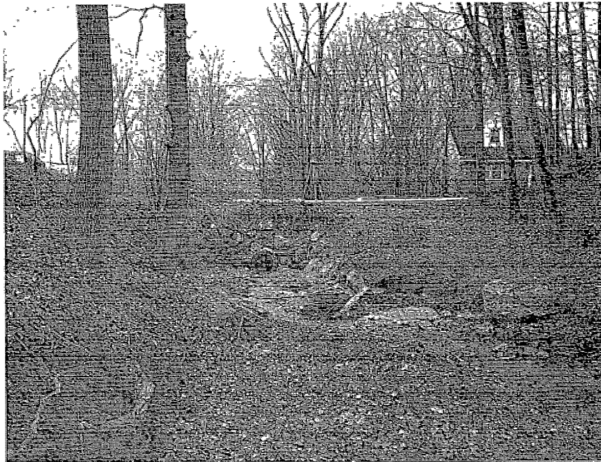
Facing downstream toward Thurston culvert in northern tributary. Culvert blocks frequently and causes flooding on Thurston. Proposed right sizing of culvert to better accommodate high flows and reduce downstream velocities.
