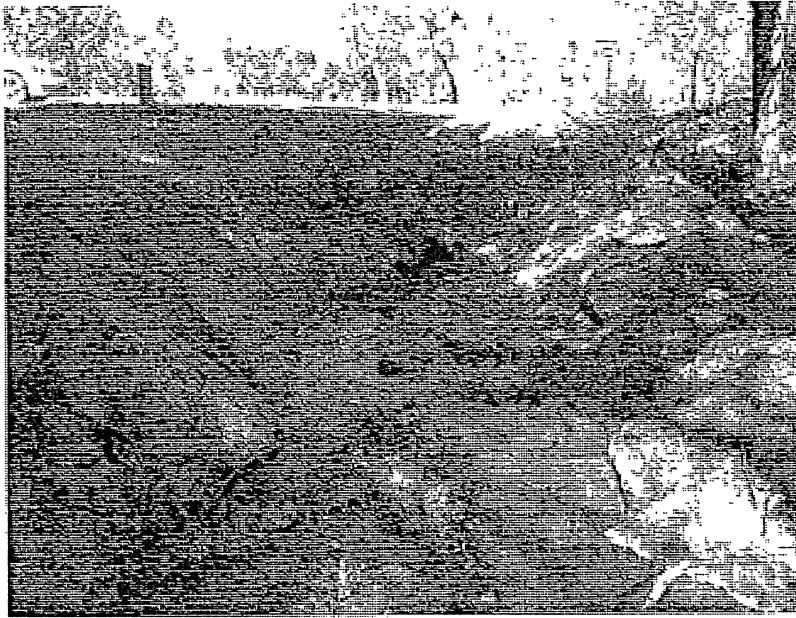
Facing downstream toward Thurston Culvert on Southern Tributary. Note blockage at invert. Approximately 0.5' of sediment is accumulated in the pipe. The pipe frequently clogs and floods the road. This combines with the blockage and flooding from the northern tributary to make Thurston impassible for residents and motorists. Proposed right sizing this culvert.
