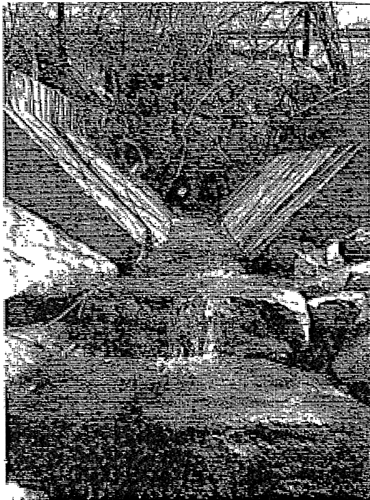
Downstream exit of Oneida Street culverts through concrete chute. Proposed replacement of pipe with right sized structure and grade controls. Upstream start of proposed Step Pool Storm Conveyance project to Sauquoit Creek.
