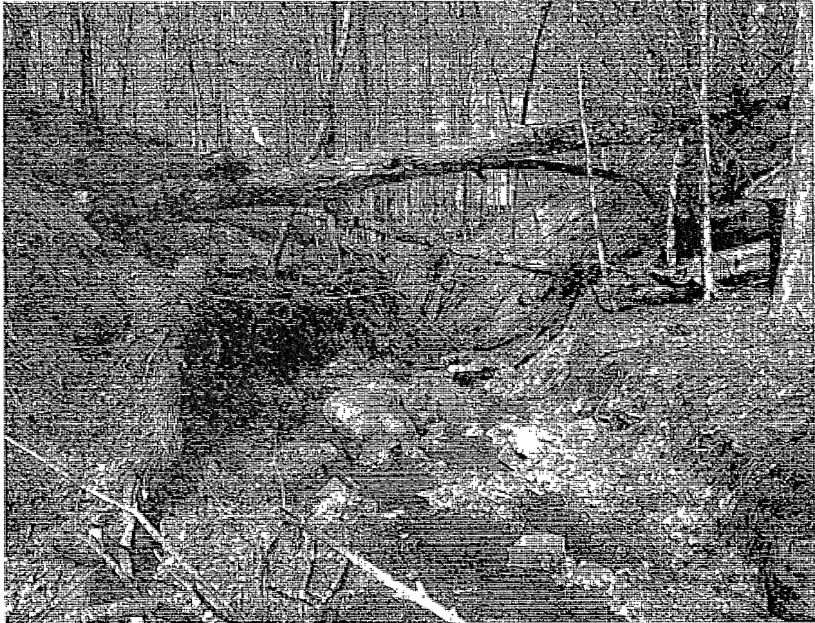
Erosion in Southern Tributary.
