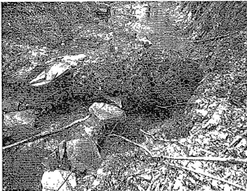
Gabions installed by the Town at an unknown time have held up well considering the storm events. Where access is possible, replace these with more robust rock structures.
