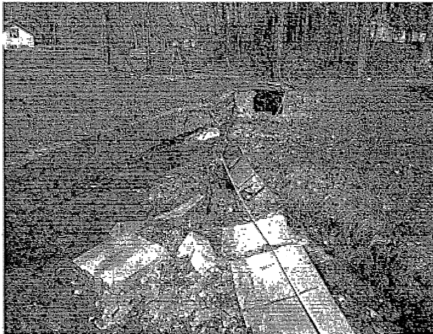
Facing downstream in armored channel that is undersized and failing. Proposed right sizing of channel to bankfull dimensions and removing the downstream culvert which is rusted through at the base.
