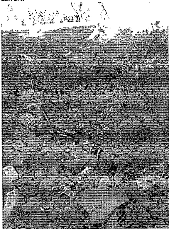
Facing downstream toward catch basin over Thurston culvert on Southern Tributary; note scour.
