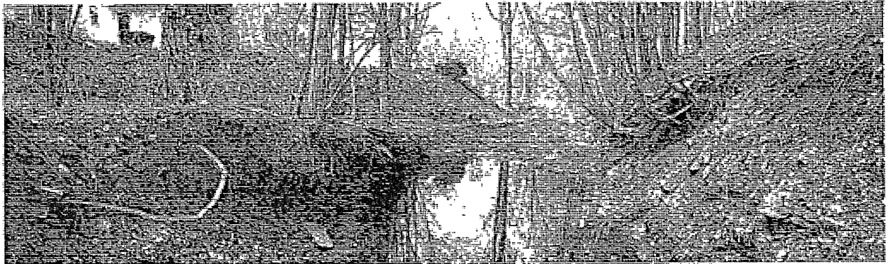
Facing downstream in northern tributary on upstream side of Thurston; erosive banks are undermined.
