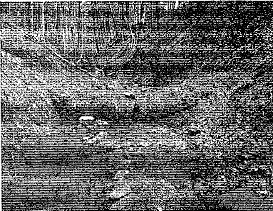
Gabions installed by the Town at an unknown time have held up well considering the storm events. Where access is possible, replace these with more robust rock structures.
