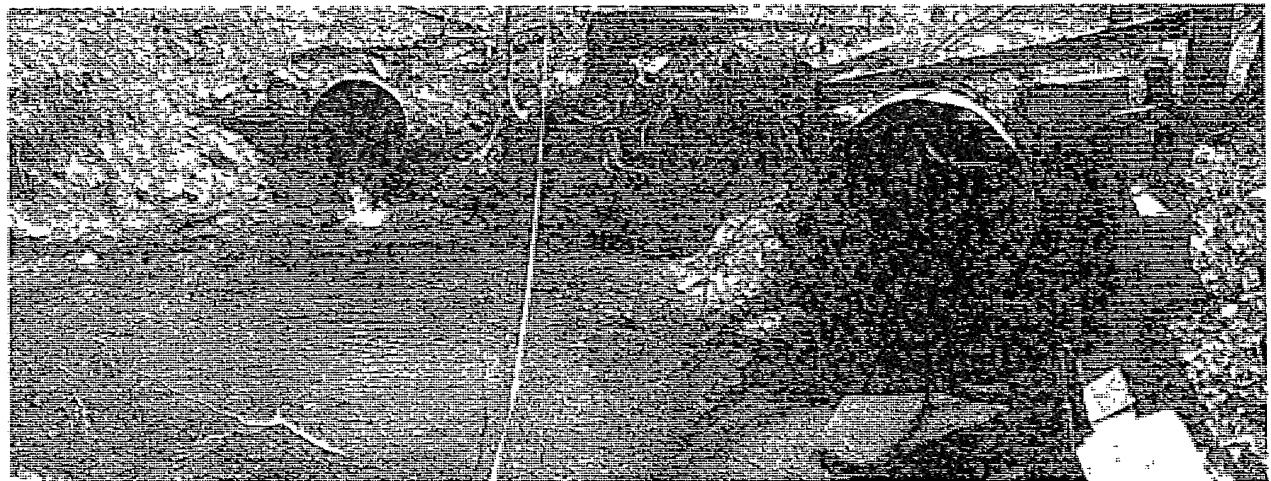
Facing upstream at Northern (left) and southern (right) corrugated metal culverts that are rusted at their bases. Proposed culvert removal and daylighting streams to proper dimensions.
